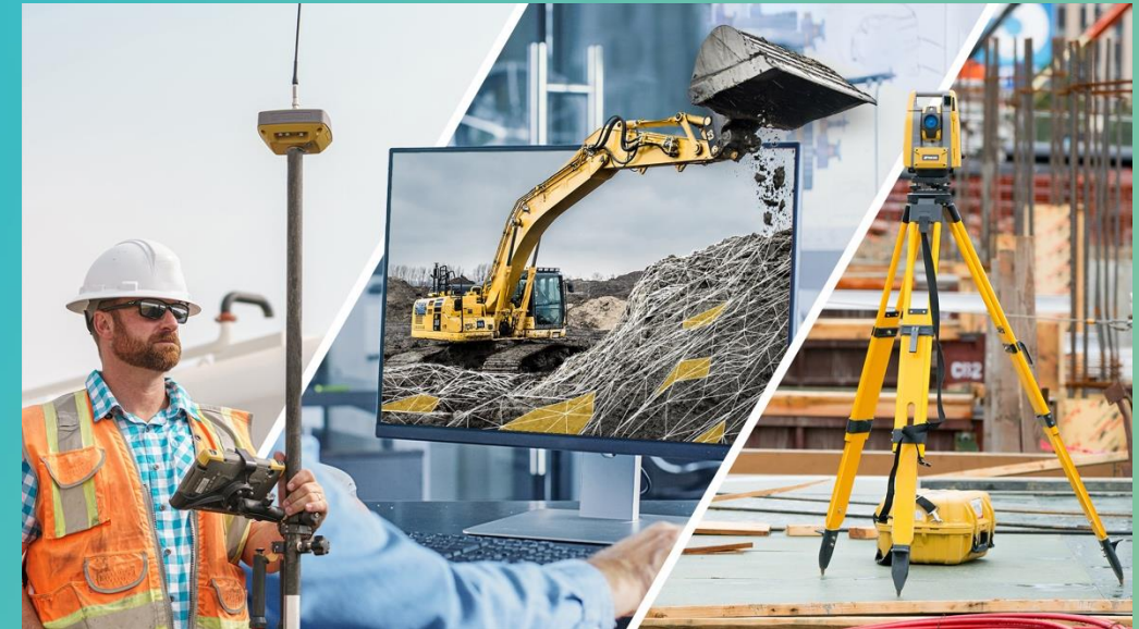
© Topcon Positioning Systems, A 5G Campus Network connects humans and machines at a construction site.
